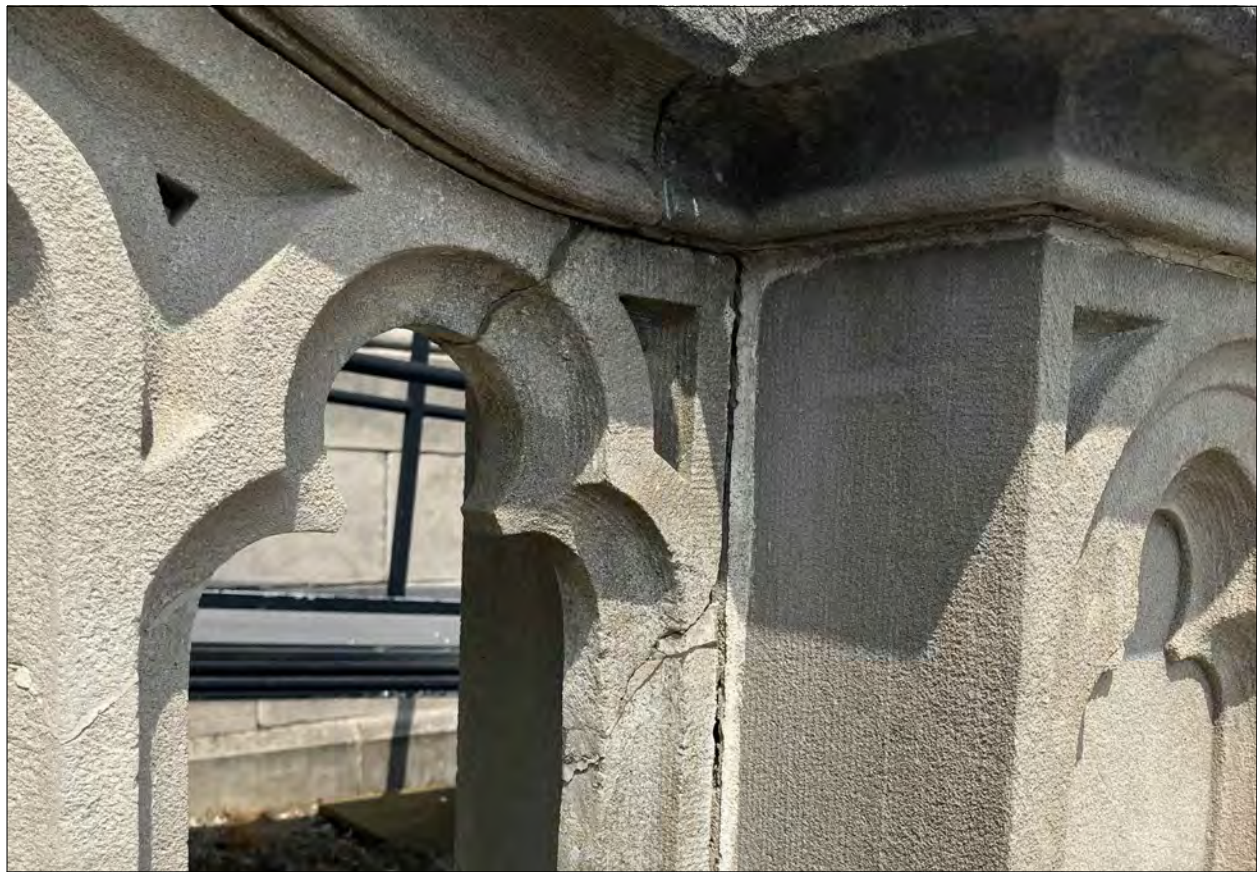
O2: EXISTING DAMAGE
