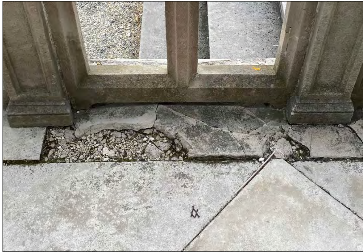
O3: EXISTING DAMAGE
