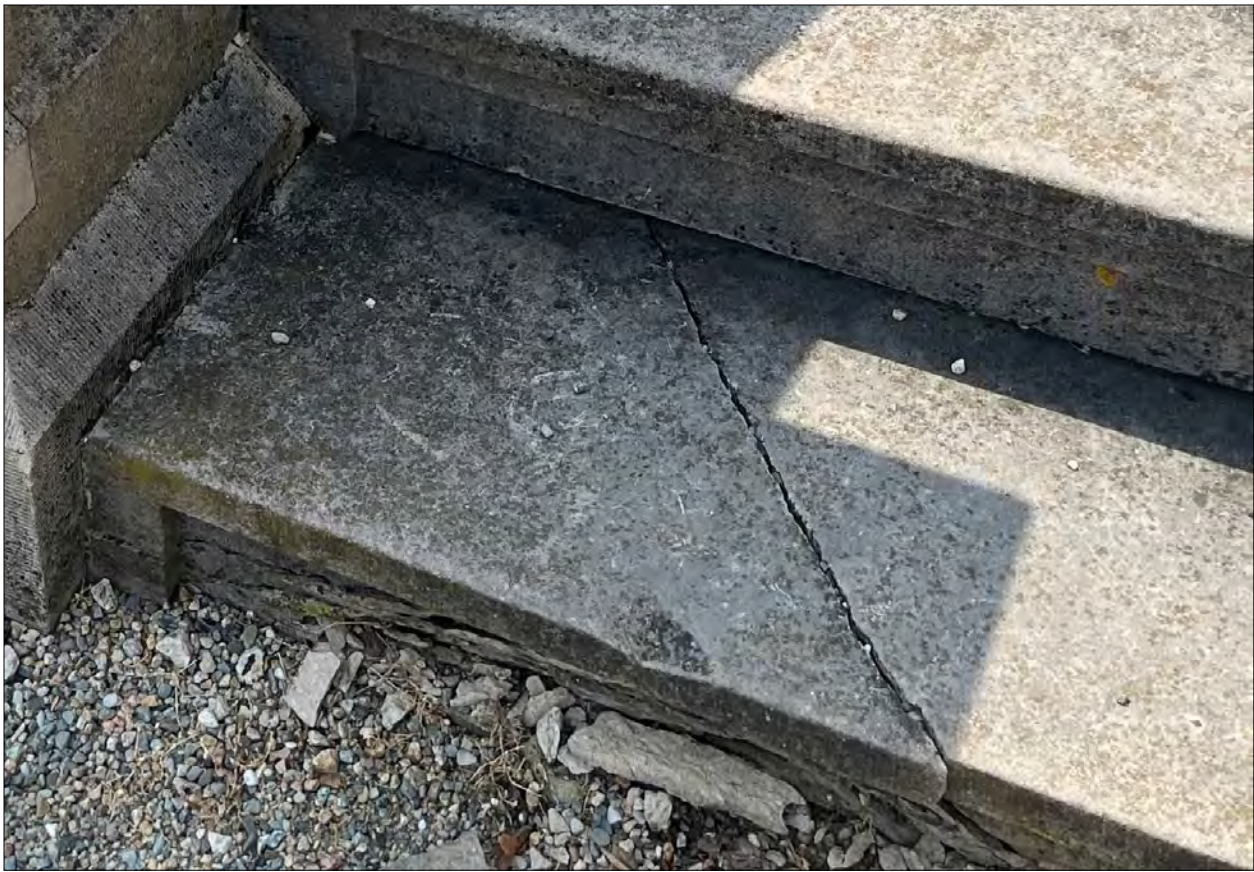
O4: EXISTING DAMAGE
