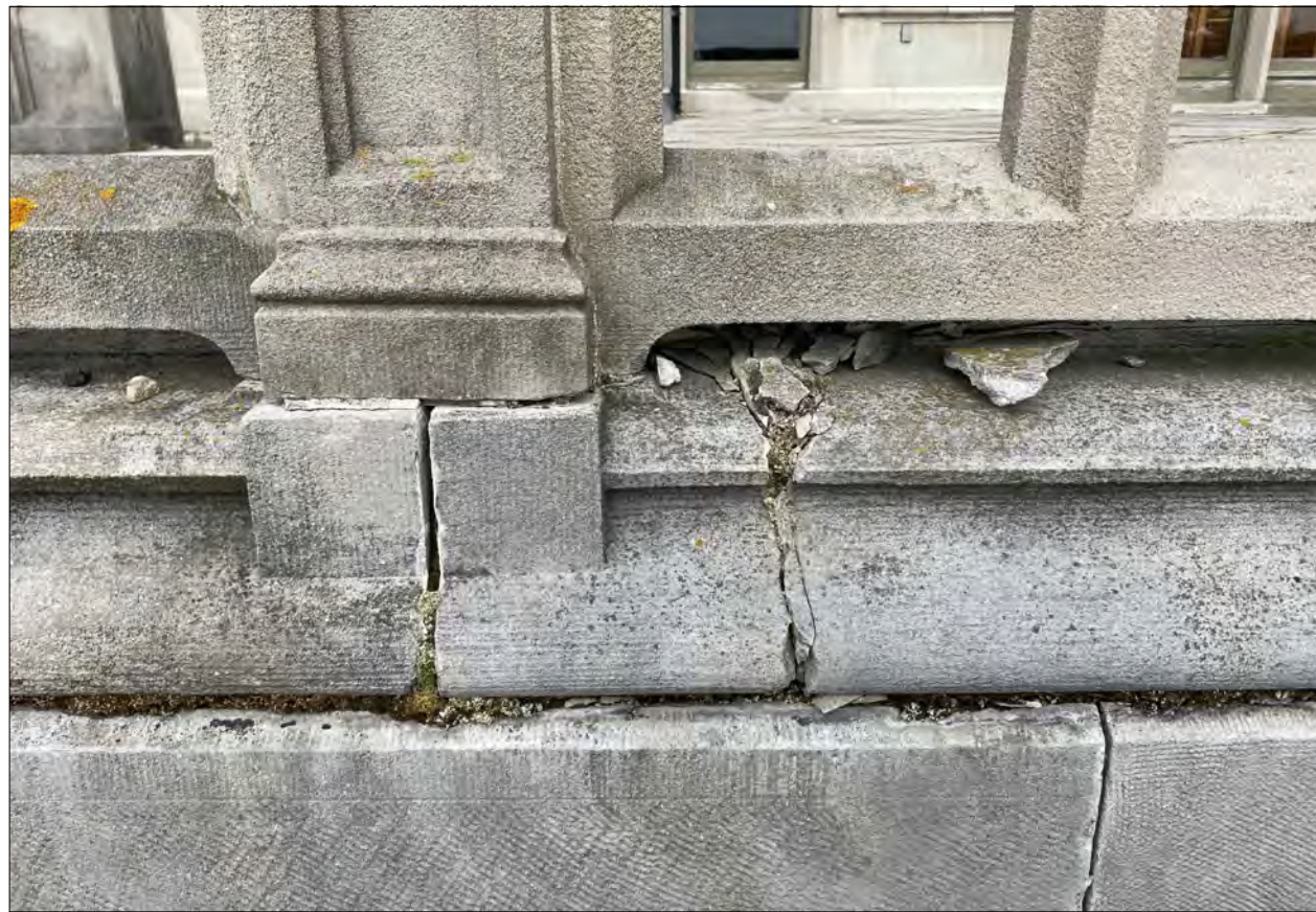
O1: EXISTING DAMAGE
