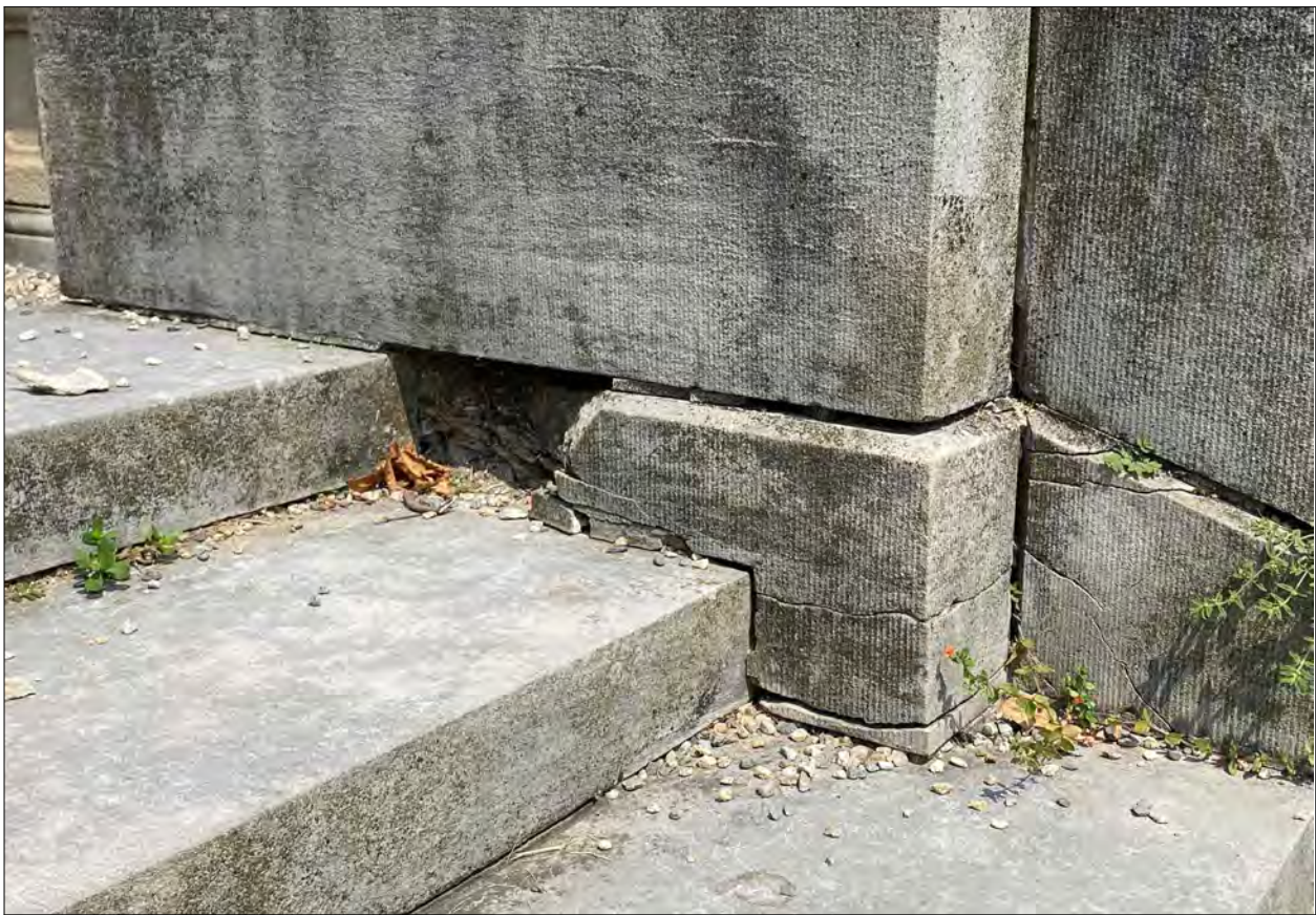
O2: EXISTING DAMAGE
