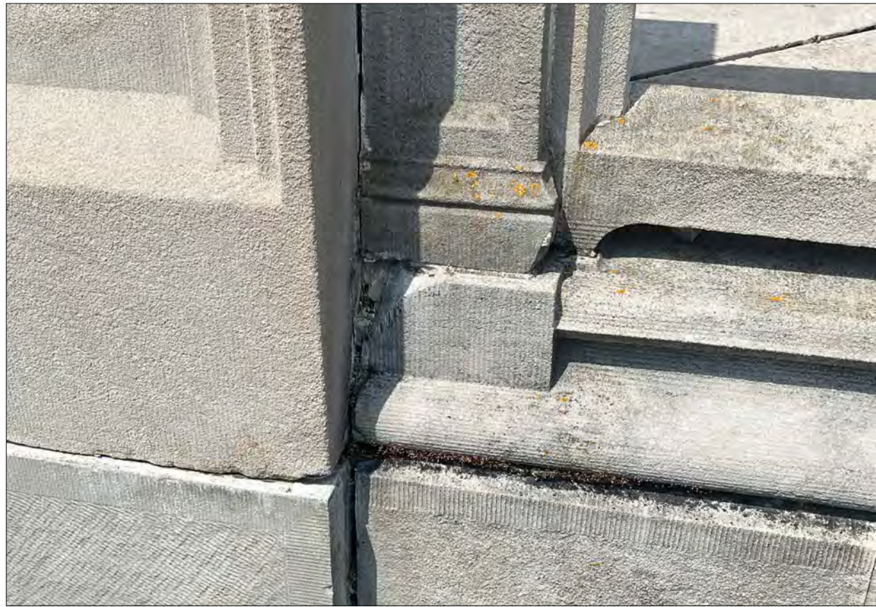
O3: EXISTING DAMAGE
