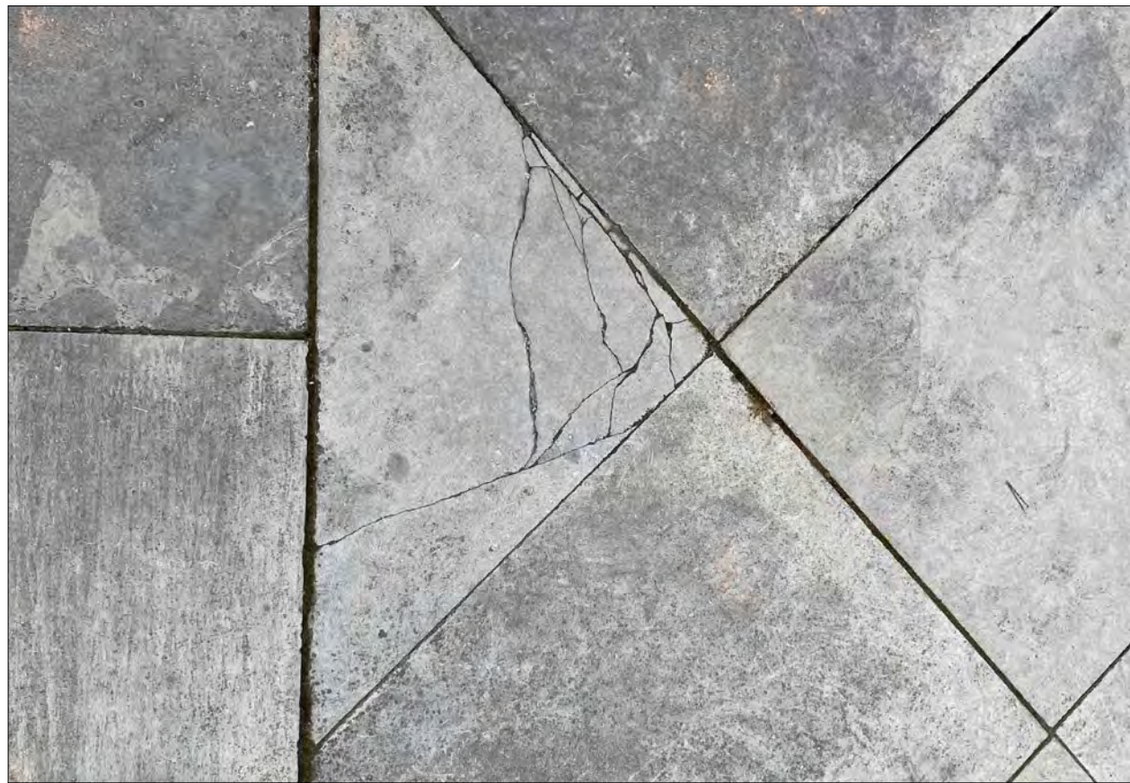
O1: EXISTING DAMAGE
